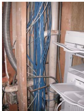
The result of water damage that occurred at the courthouse over Easter weekend.
